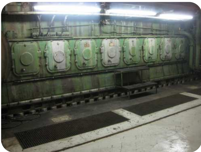
Overview of engine mounted on SKF Vibracon chocks on a concrete foundation.
