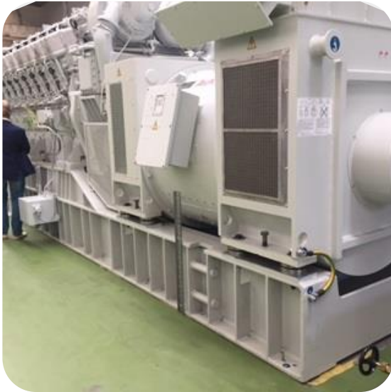
Generator of generator set mounted on SKF Vibracon chocks.
